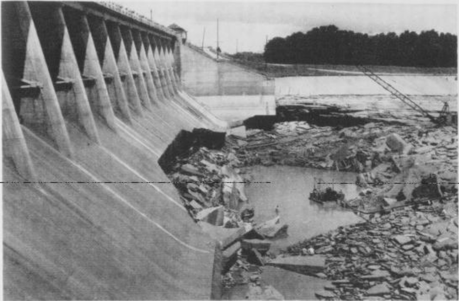
FIG. 20-4. Damage due to scour and uplift pressure at Waco Dam, Texas. (Courtesy of Waco City Water Department.)
