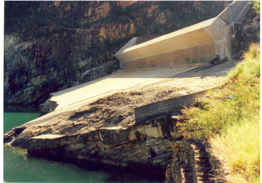
Backcutting scour progress at Estreito dam, Rio Grande, Brazil [source: CBDB, 2006]
