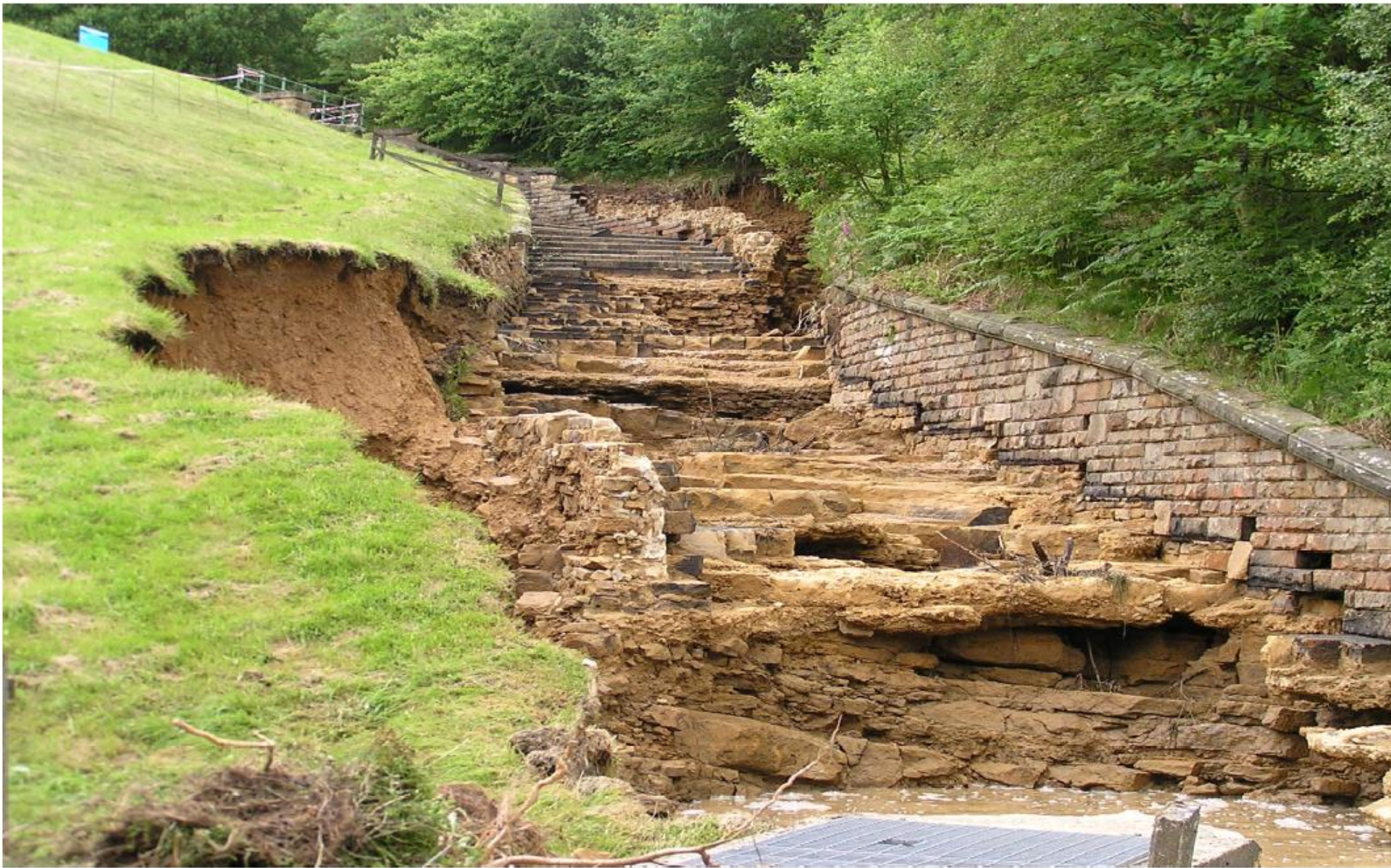
Figure 7 - Damaged spillway at Boltby in 2005
