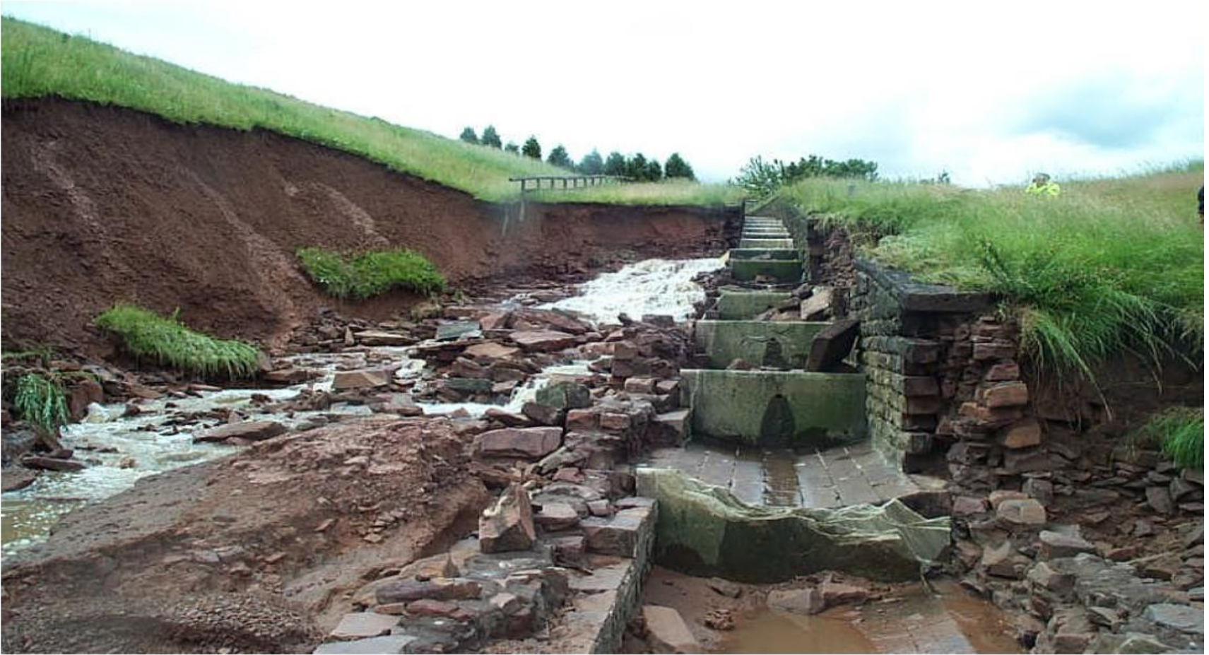
Figure 3 - Scour hole photographed on Tuesday 26 June, 2007
