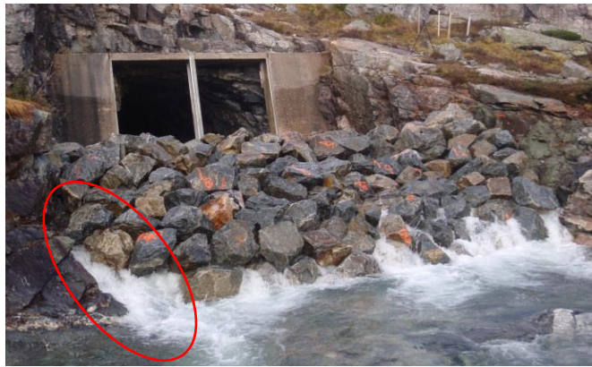
Figure 8, Red ellipse shows where two stones were dislodged from the riprap during overtopping.
