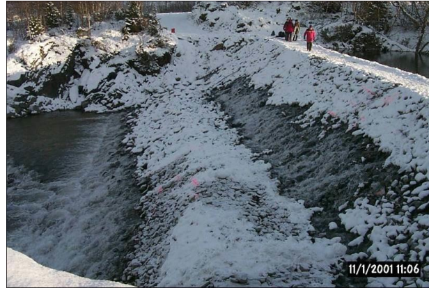
Figure 2, Downstream erosion on rockfill dams, Photo: EnFo
