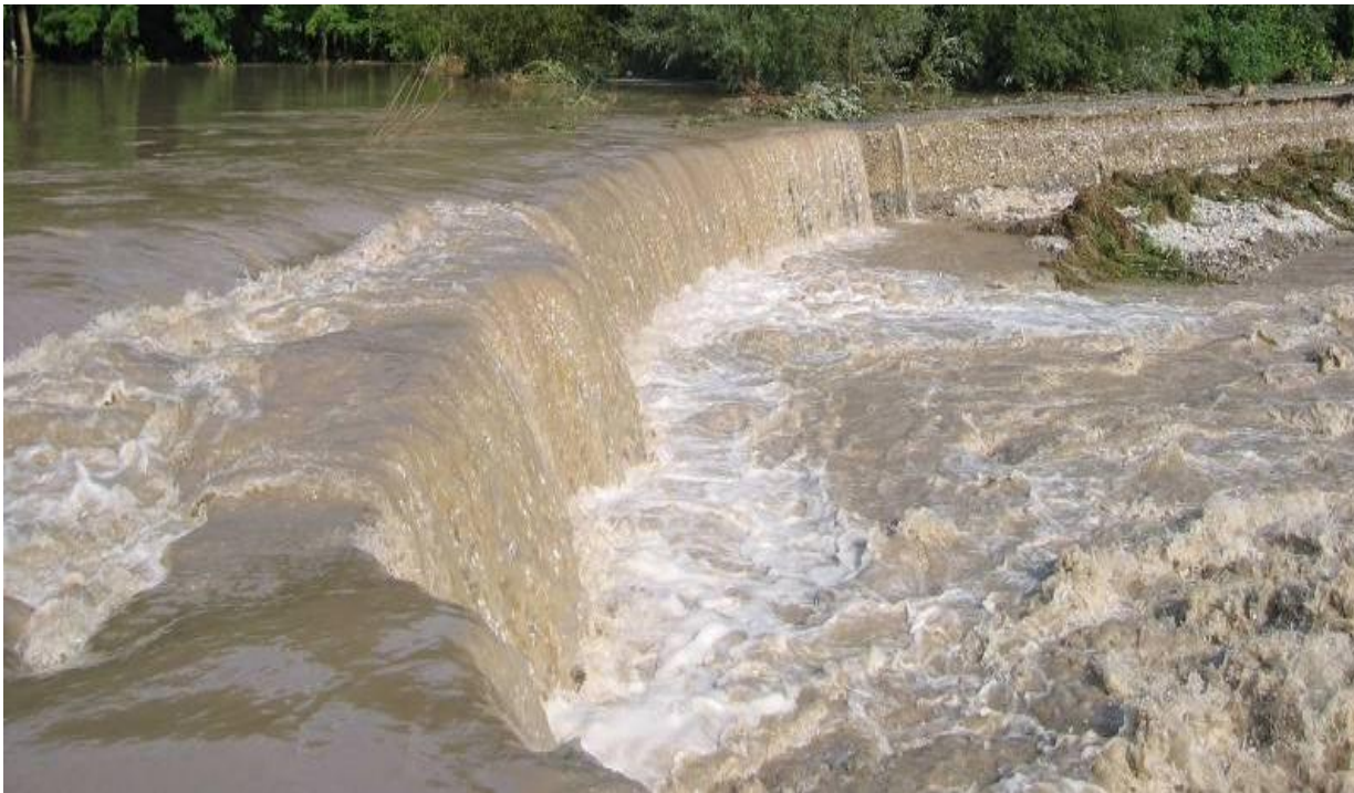
Unreinforced sealing core with erosion of the embankment, flooding 2005 Iller Water Agency Kempten
