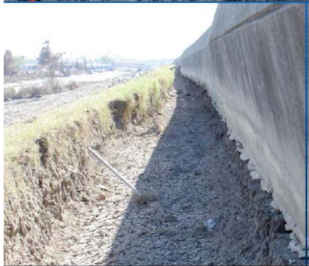
Figure 22. Example of breach along IHNC (east side) from overtopping and scour (top) and scour behind adjacent section that did not fail (bottom).
