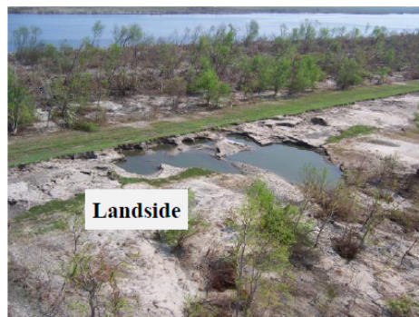
Stage D: Overtopping erosion at Bayou Dupre in St. Bernard Parish
