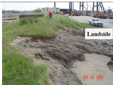
Stage B: Headcut erosion along the IHNC
