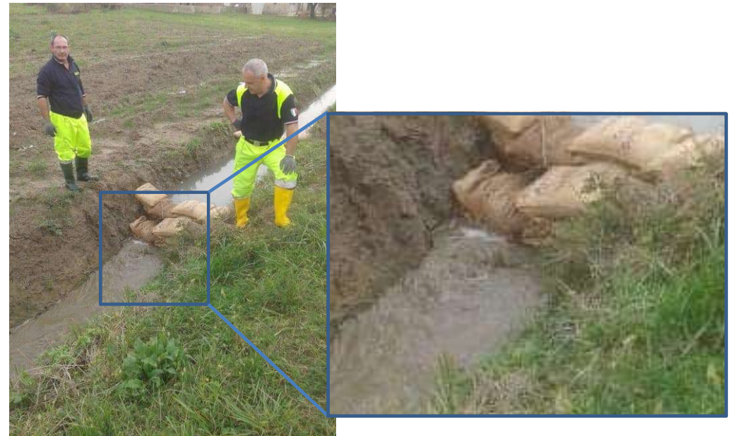
Picture of the sand boil at the initial stage of the reactivation
